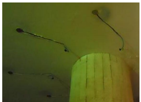
Furrows of the electrician after the painter did his job
